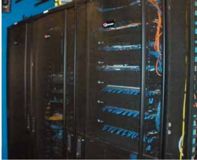
Siemon's VersaPOD cabinets provide space savings and thermal efficiency in the main equipment rooms.
